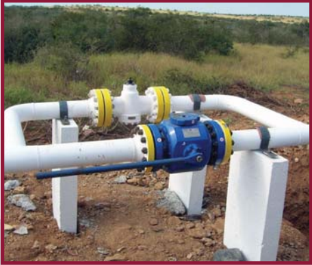
6" 600 ANSI with 6" bypass line, Tamaulipas, Mexico
