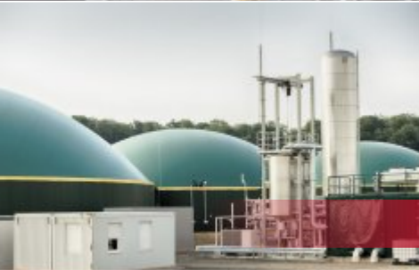
Flare gas and vapour recovery system
